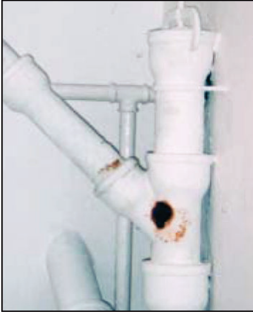
Rust is an indicator that condensation occurs on this drainpipe. The pipe should be insulated to prevent condensation.
