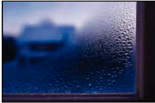
Condensation on the inside of a windowpane.
